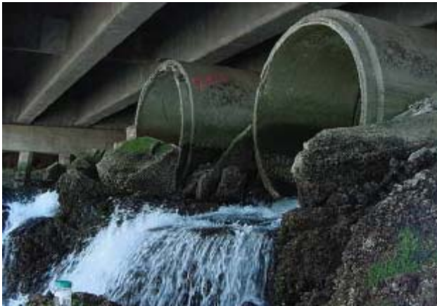
Figure 3. Twin eight-foot diameter outfalls that discharge stormwater into the Thea Foss Water Way (Source: City of Tacoma 2006).
