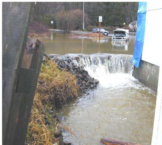
Figure 2. Flooding at Old Belfair Highway near Gorst in Kitsap County. Photo courtesy of Dave Dickson, Public Works assistant director of Kitsap County, WA.
