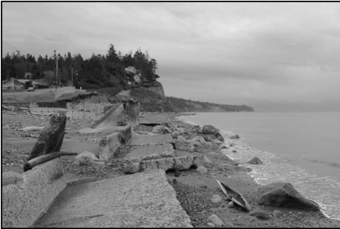
Broken concrete bulkhead on West Beach Road, Whidbey Island. | Photo by Marsha Engel
