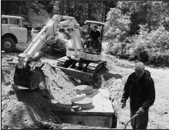
Workers retrofit an existing septic system on a Hood Canal property. | Photo by Terry Hull
